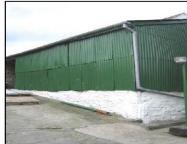
Storage facilities, 22 weeks, SR 170 kgN/ha, minimal soiled areas , Guttering and downpipes, well managed facilities
